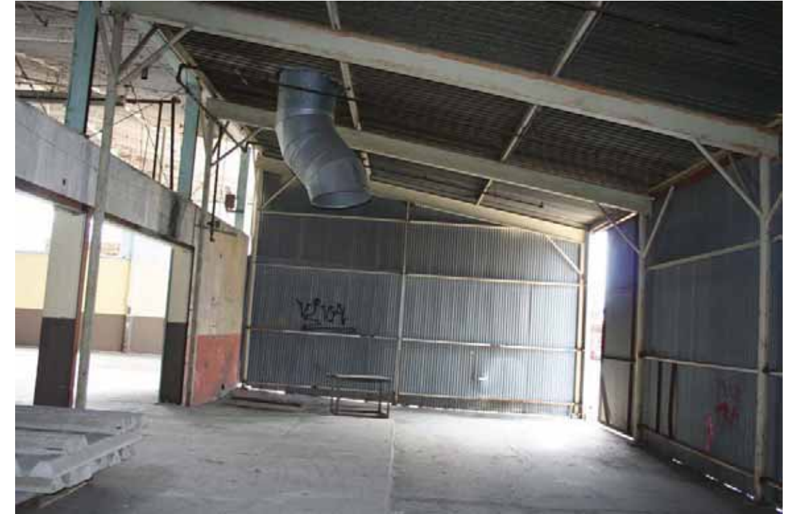
Building 513 - Ancillary Building Associated With Building 156, Interior, facing South with Building 156 to the left, San Diego, California, October 2009.
