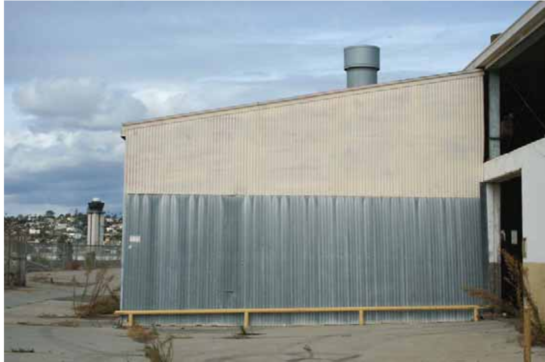
Building 513 - Ancillary Building Associated With Building 156, South Elevation, San Diego, California, October 2009.
